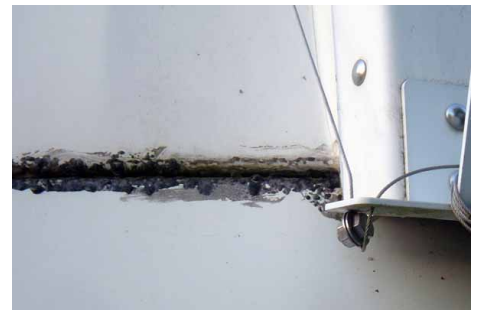
Note how the epoxy seams had turned black and rock-hard and ugly. After disassembly and trucking it back to Barrington, the first step was a much needed power wash.
