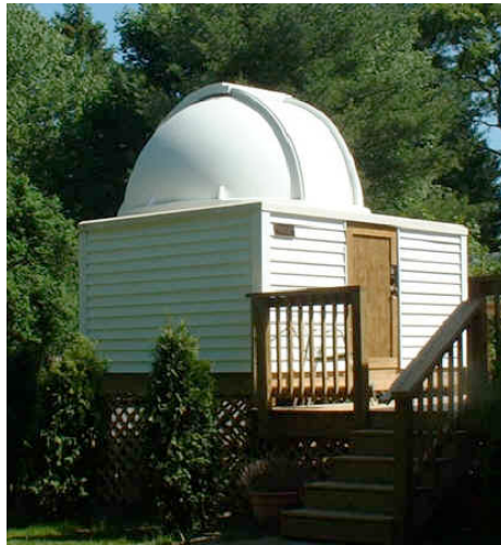
And finally railings are installed on the stairways to provide full compliance with local codes. The observatory was blessed by the Building Inspector on 19 Jan 07.
