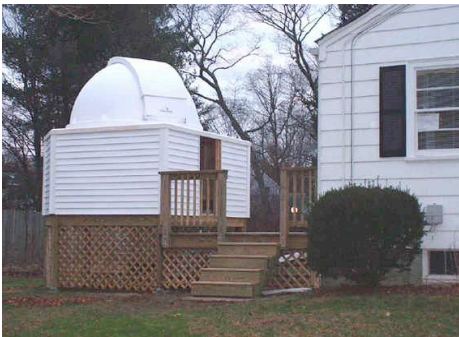
Here's the status as of Dec 12th. Front stairs finished. Front railing finished. Skirt partially complete. It's starting to look real.
