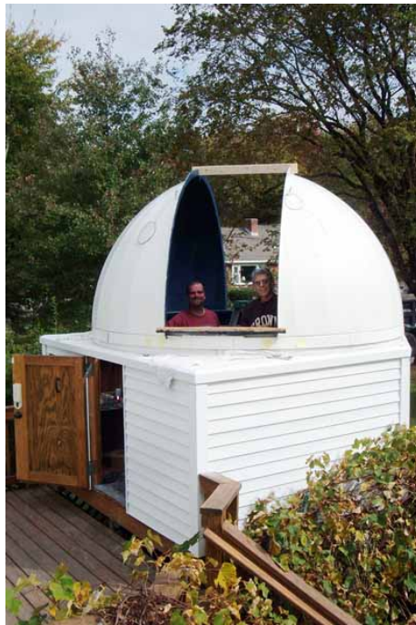
The two hemispheres are now up and positioned with spacing timbers to establish precise shutter spacing.
