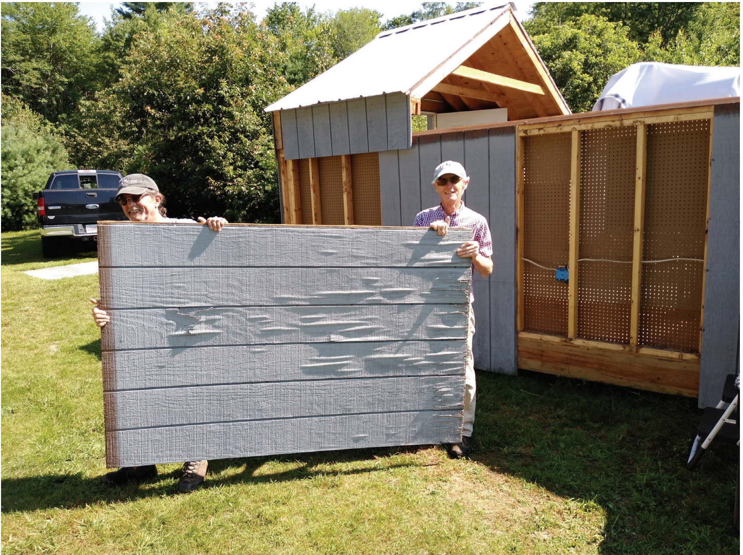
Work In Progress: Tom Thibault (left), Jim Crawford (right) and Jim's son, Brian, have been replacing several of the T-111 panels on the roll-off sheds for the Meade 12 and 16 inch SCTs. During these sessions the trustees have also been present to help and regularly mow the observatory's "astro" turf.
